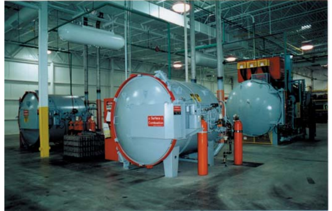
furnaces at manufacturing
